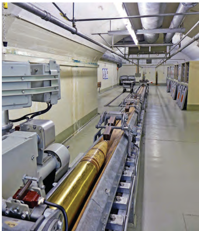
Fort Dailly: The ammunition carousel at the foot of the vertical shaft to the turret Fort Dailly: The shell conveyor for T1, viewed from near the carousel, with the ammunition preparation area at the far end
